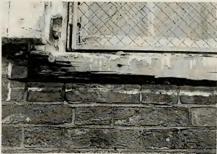
Figure 28 Wood Window Sill Deterioration, 1998 Photograph by Author
